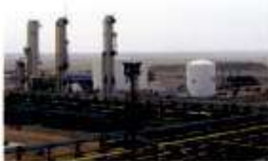
Water purification station
